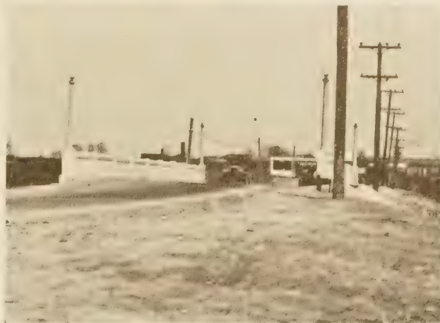
FIGURE 17.—SETTLEMENT OF ROAD AT BRIDGE APPROACH DUE PRIMARILY TO THE CONSOLIDATION OF THE THOROUGHLY SATURATED UNDERSOIL
